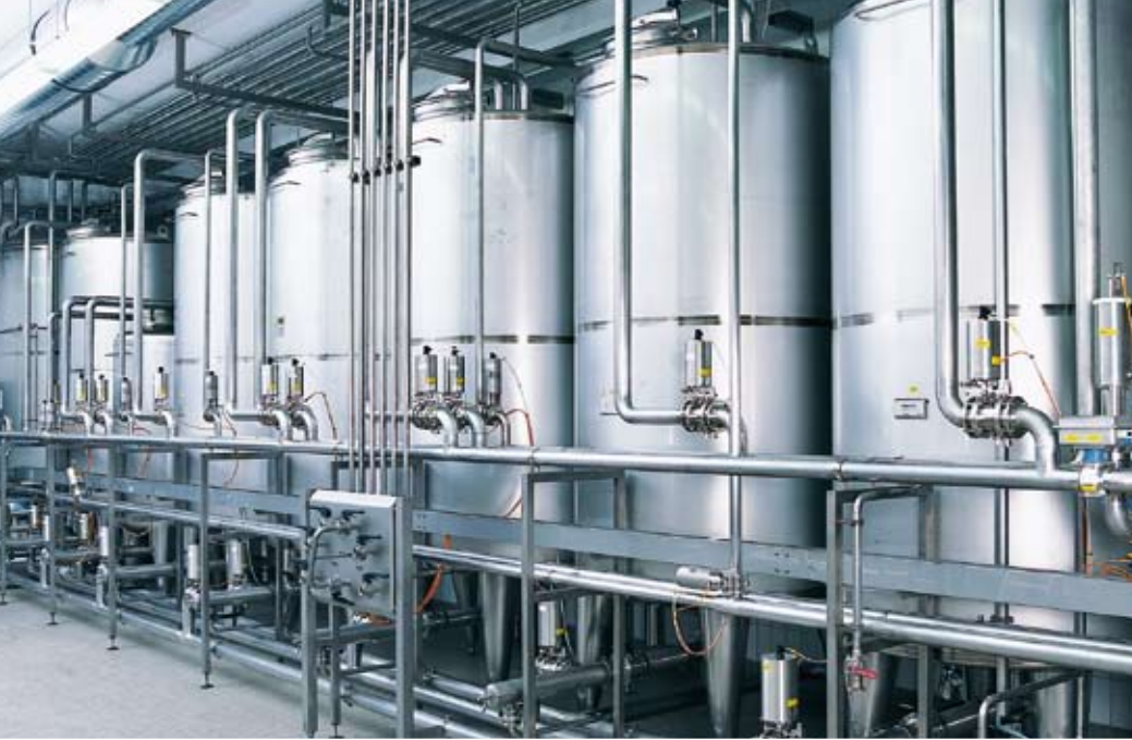
CIP tanks, Auer Bräu AG, Rosenheim/ Bavaria
